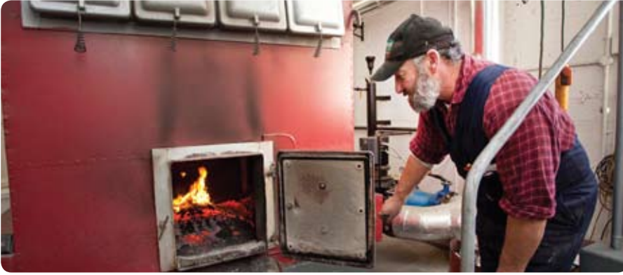
Geoff Parkin, Property Manager, checks the converted boiler.
