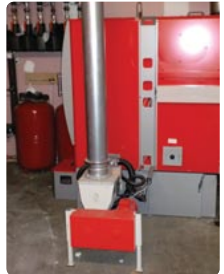
The wood chip boiler operating the University’s Property Services division.
